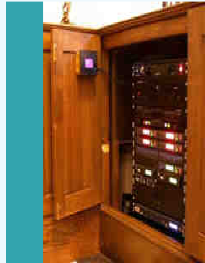
Equipment rack with mains power conditioning unit at the top
