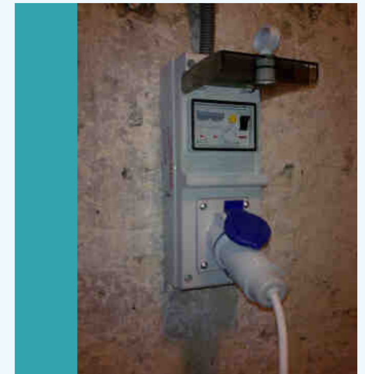
RCBO protective 16 amp outlet
